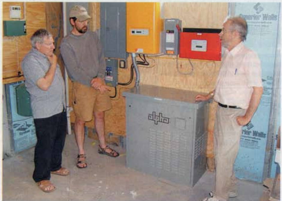
HARNESSING THE SUN: Hundredfold Farm residents Joel Plotkin, left, Bill Hartzell, center, and David Pierce discuss how each house in the project harnesses the power of the sun to create electricity. Roof panels generate electricity that flows through an inverter and battery pack before becoming common household electrical current. Power generated by the unit is used to reduce the homeowner's electric bill. Any excess power is "banked" for which the homeowner will receive credit at year's end.
